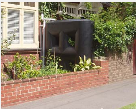
Residential water tank
