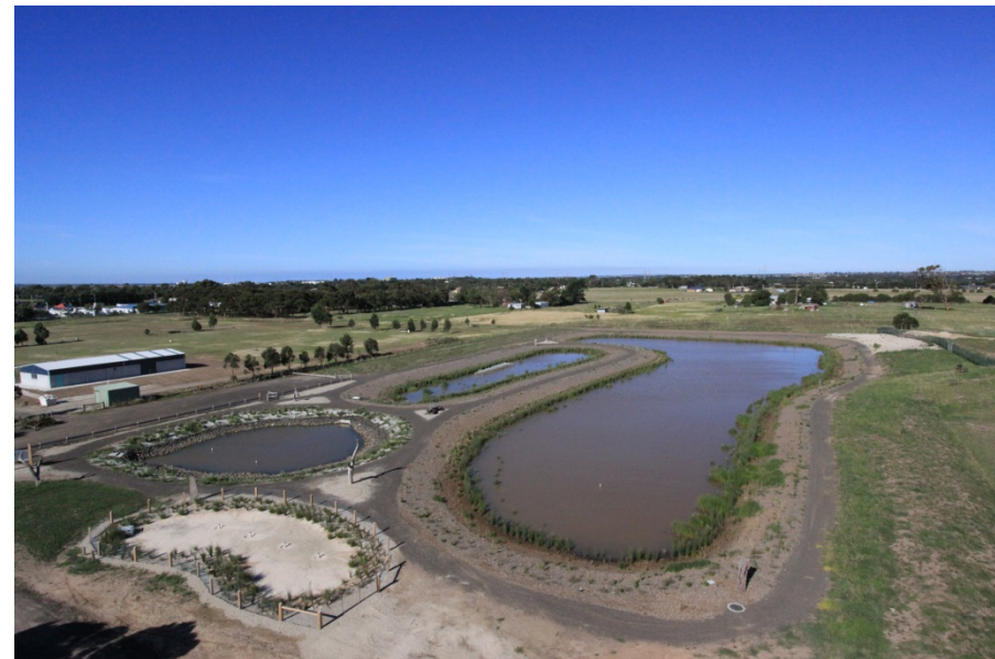
Grinter Reserve - Construction of wetland February 2011 Image courtesy of the City of Greater Geelong
