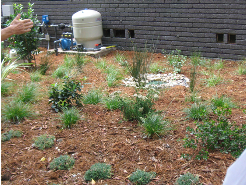
Figure 11: Property Drain “Pop-up” within a rain garden, Santa Monica, USA
