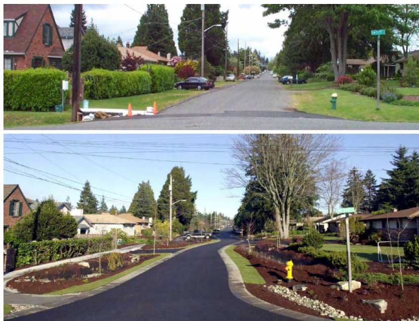
Figure 10: A before and after shot of a reconstructed roadway to incorporate swale drains with curve-linear road alignment (Mills, 2008)
