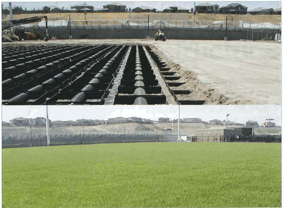
Figure 4. Subsurface stormwater storage for a sports field, USA.
