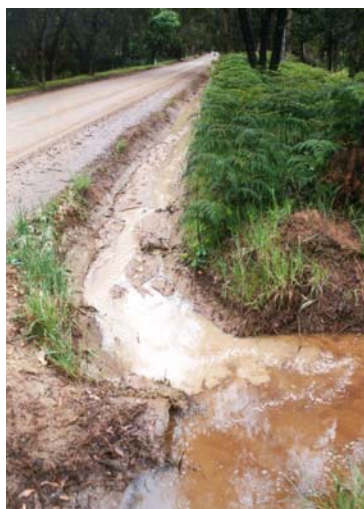
Photo 5: A table drain along an unsealed road following rainfall.
