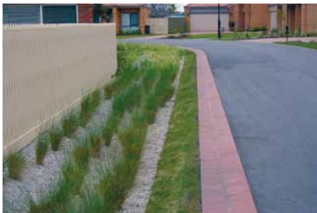
Figure B-1: Bioretention Swale
