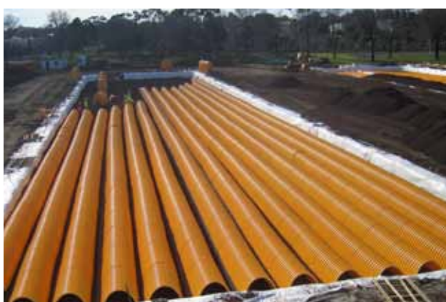
Figure B-10: Stormwater harvesting Source: Melbourne Water.
